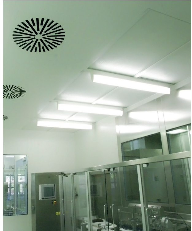
TDL Lighting system
